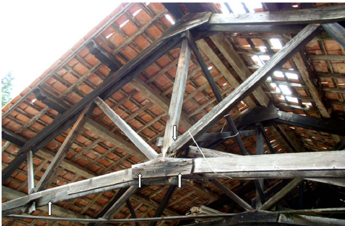
Image 1. The warehouse in the Nineties. Damages on the first truss: the bottom chord was broken (left arrow), the joint "N" was severely disconnected with end tie rod badly decayed and bolts evidently bent (central
