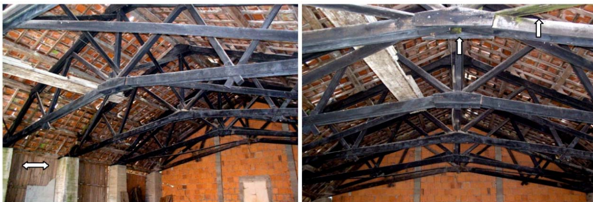
Images 2-3. The warehouse in the nineties. The green biofilm is present and visible on the roofing, on two columns (image 2, white arrow) and on the plank converging on joint named "N" of the second truss (image 2, white arrows).
