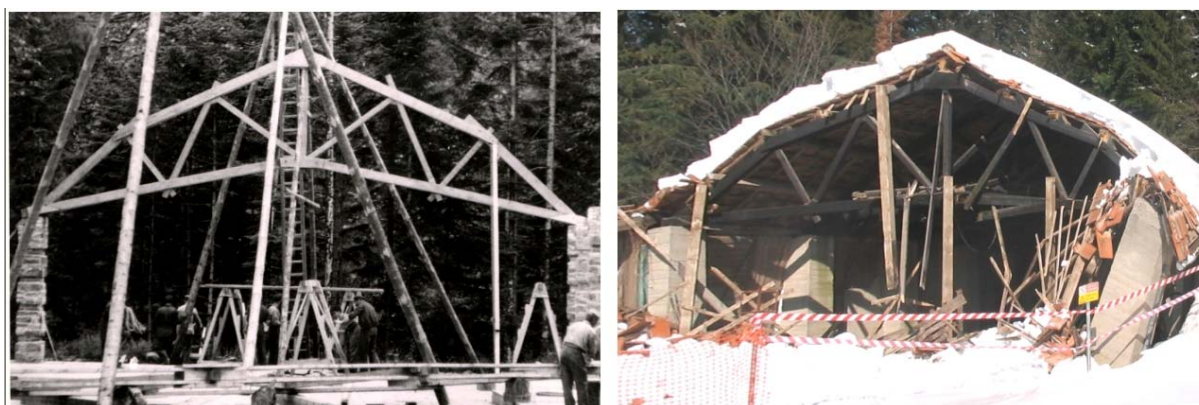
Images 11–12. Comparison between two symbolic instants of the shelter life: the first truss erected, reproduced in an original photo, dated 1952, and the warehouse without the first truss, collapsed under the snow load, in 2005.
