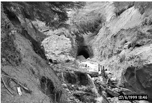
Figure 8. Same water outlet after water outburst
