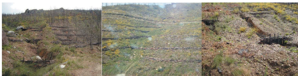
Figure 9. Barriers in burned areas (in gullies and slopes) of Gerês mountain, North of Portugal, constructed post-wildfires with materials of burned trees.
