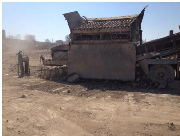
Figure 21 - Grizzly plant used to separate clay and sand from demolition debris before crushing
