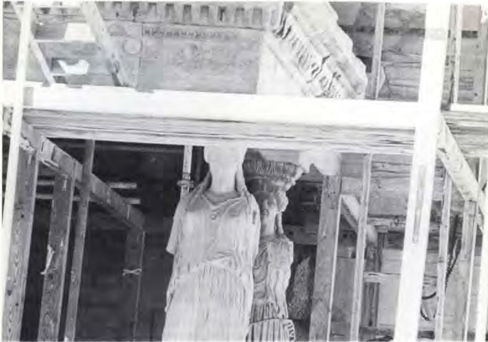
The caryatids of the Erechtheion in Athens. The scaffolding is necessary because they have been so weakened by air pollution that they can no longer hold up the temple securely. The face on the one in the front has been virtually obliterated by acid precipitation.
