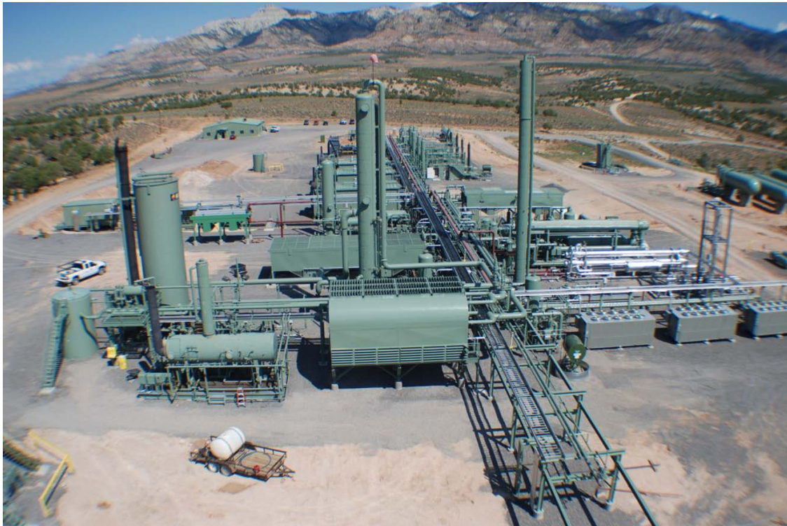
Figure 9. Natural gas processing plant (courtesy of M3 Midstream, LLC).
