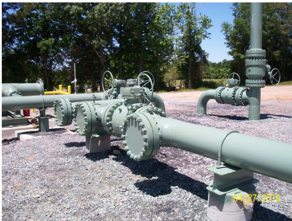
Figure 7. Gathering Line Interconnect (Courtesy of M3 Midstream, LLC)
