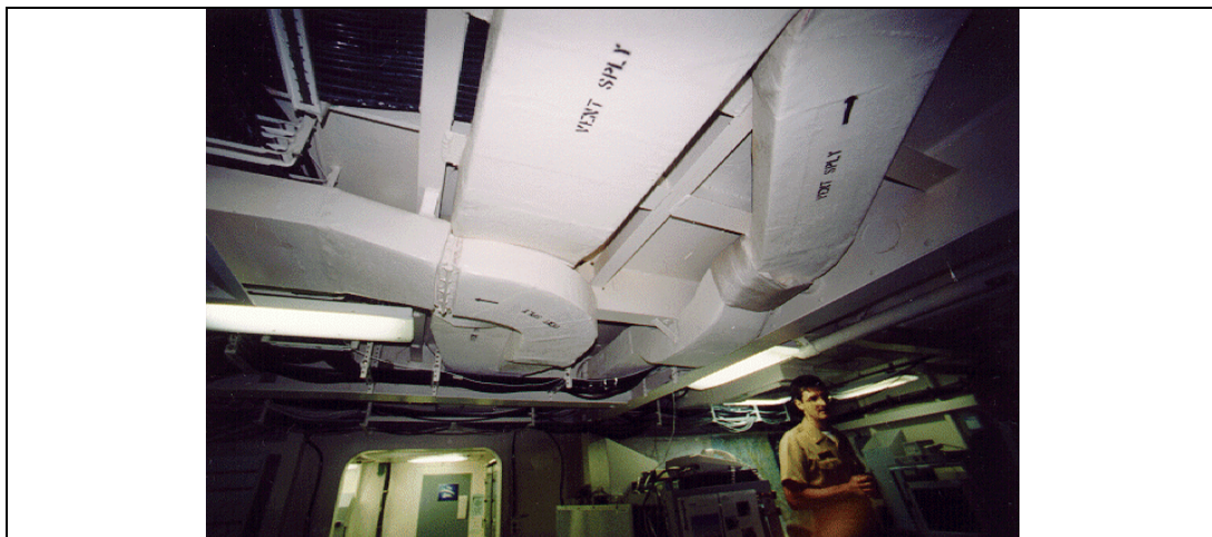
Figure 1 An example of snaking ventilation shafts in the Joint Air Operations Center aboard the USS CORONADO
