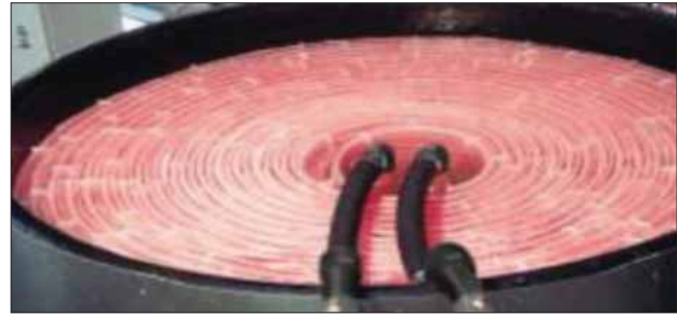
Figure 1 Internal heat exchange tubes in the Ice-bank tank.
