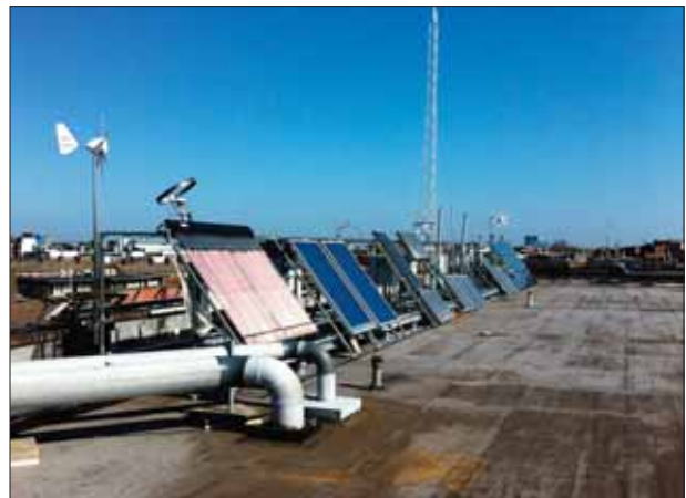
Figure 1: Renewable energy plant installed on DIT Kevin St Campus roof as part of Dublin Energy Lab (DEL) experimentation
