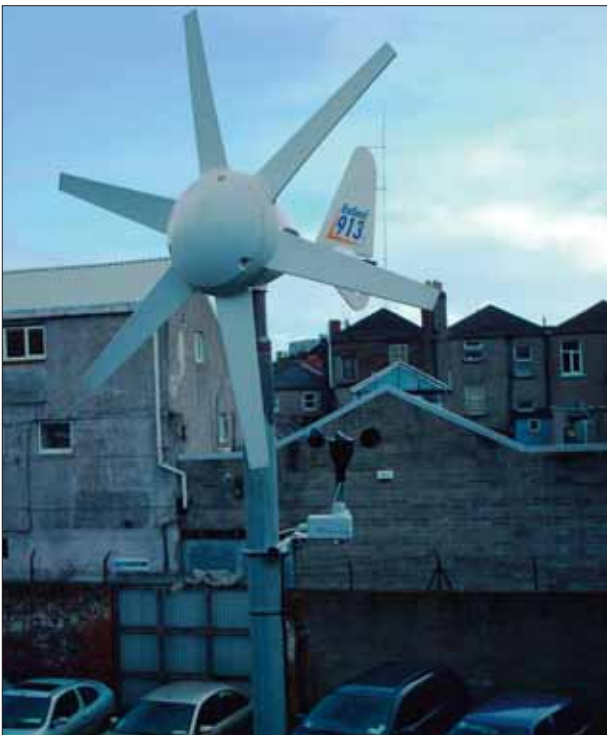
Figure 8: 220W wind charger installed in Church Lane, DIT Kevin St Campus
