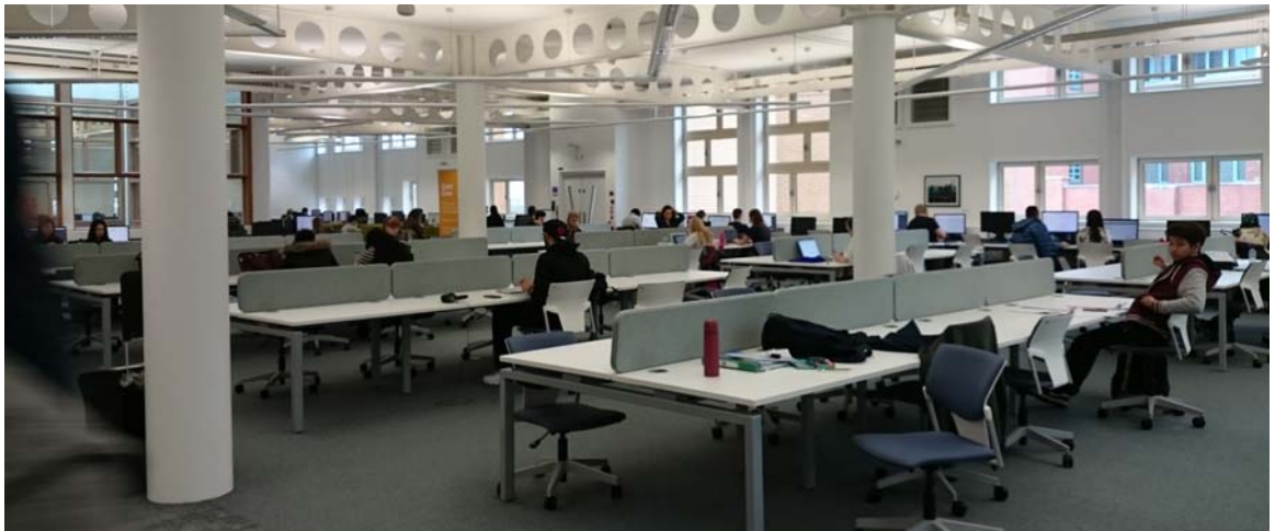
Figure 106: main library floor showing wall extract vents at high level and flat ceilings with openings cut in the web of the steel beams so that airflow is not inhibited
