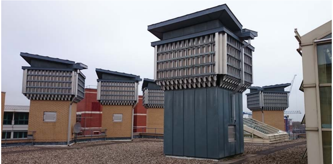
Figure 102: view of extract stacks at roof level – note blue clad stack is for top floor only
