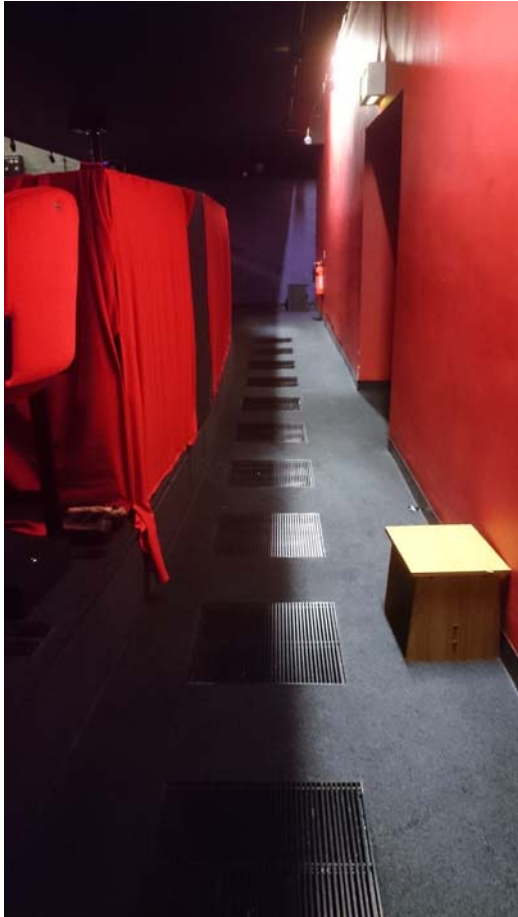
Figure 80: ventilation grills to rear of seating in the main auditorium
