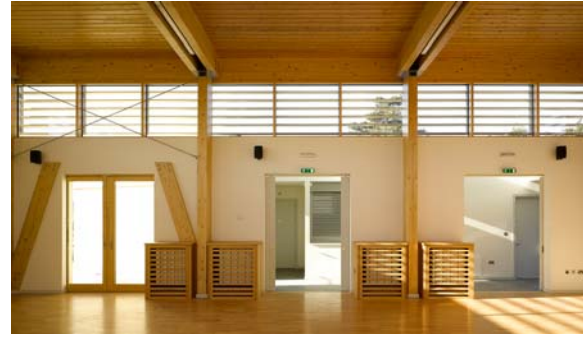
Figure 29: Air vent outlets to earth tubes, Airfield Estate, (Solearth Architecture)
