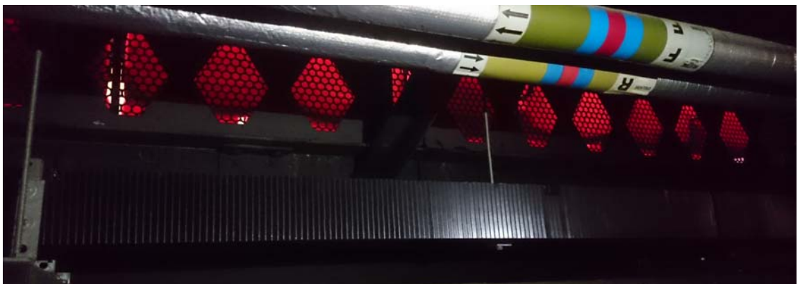
Figure 79: suspended heating elements and grills through seating to main auditorium
