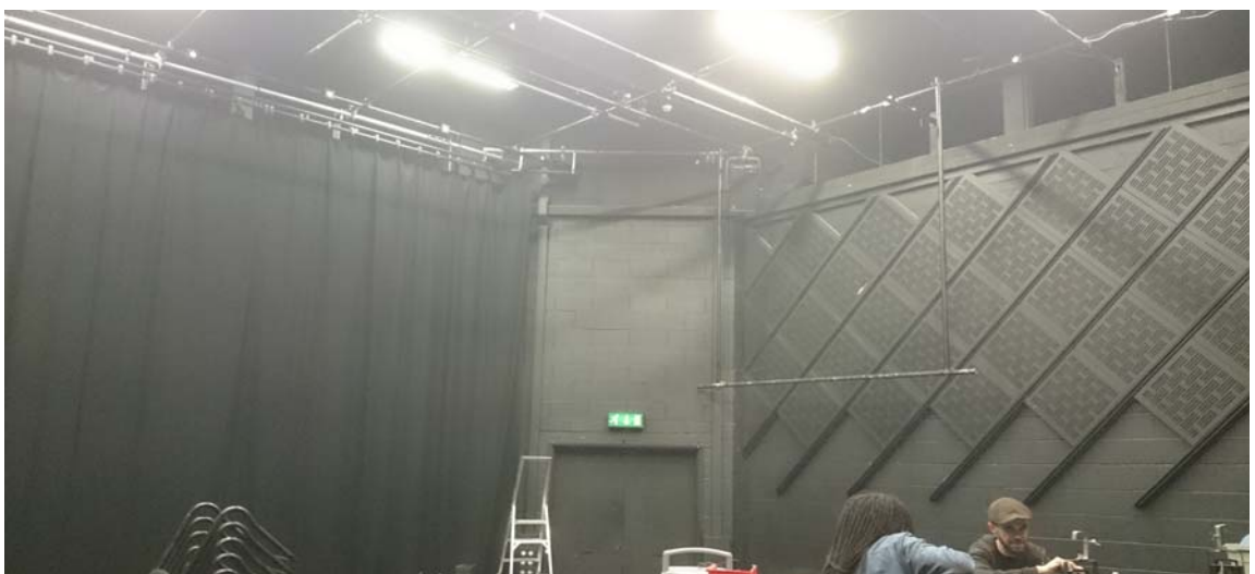
Figure 87: studio theatre space, inlet grills in floor and outlet at top of walls
