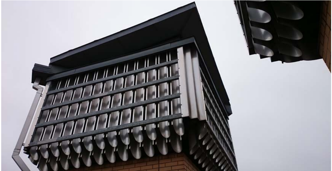
Figure 112: detail view of multi-directional extract stacks
