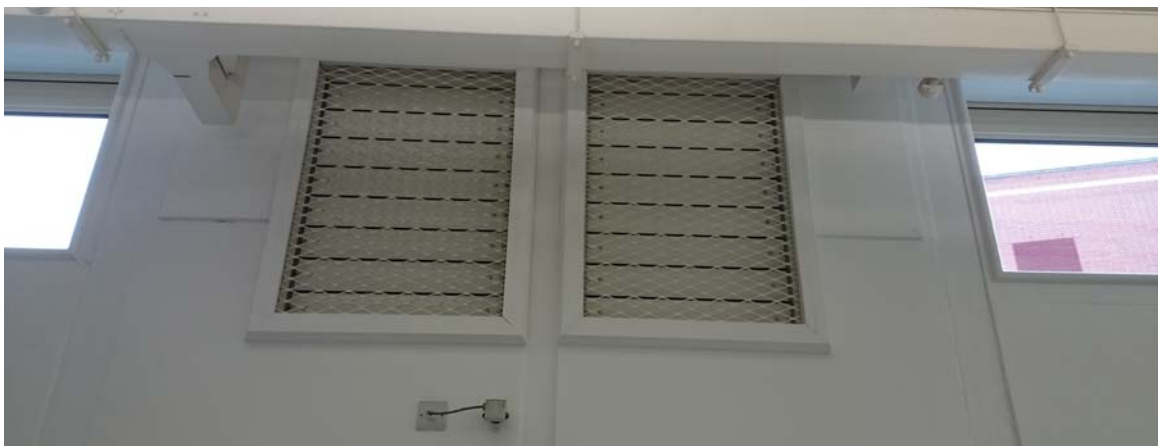
Figure 109: main library floor showing wall extract vents at high level
