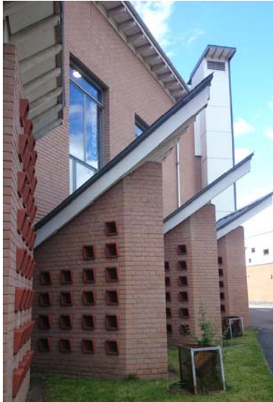
Figure 84: air intake for the foyer at ground level
