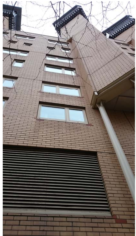
Figure 101: inlet vents at base of building
