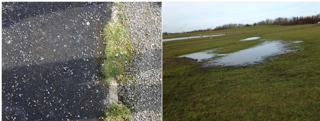
Figures 1 & 2: Photograph of broken glass (left) and waterlogged ground (right) in Darndale Park.
