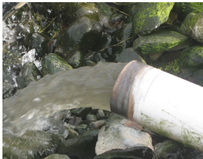
Figure 31 Inlet pipe to Horizontal flow bed, from secondary vertical beds.
