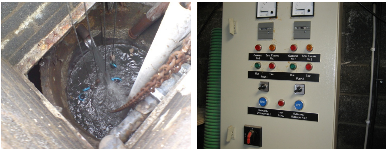
Figure 13 Pump Sump and Control Panel
