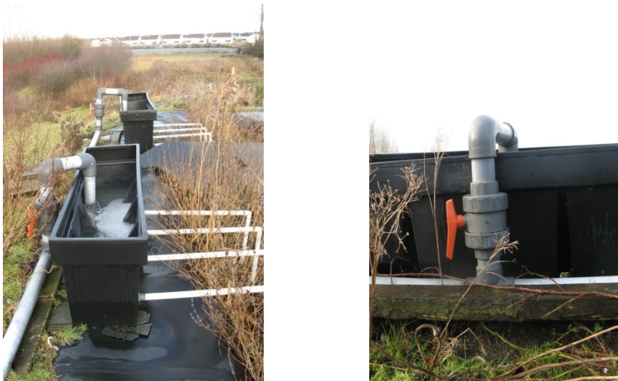
Figure 14 Primary vertical beds showing inlet pipes, valve and distribution pipes
