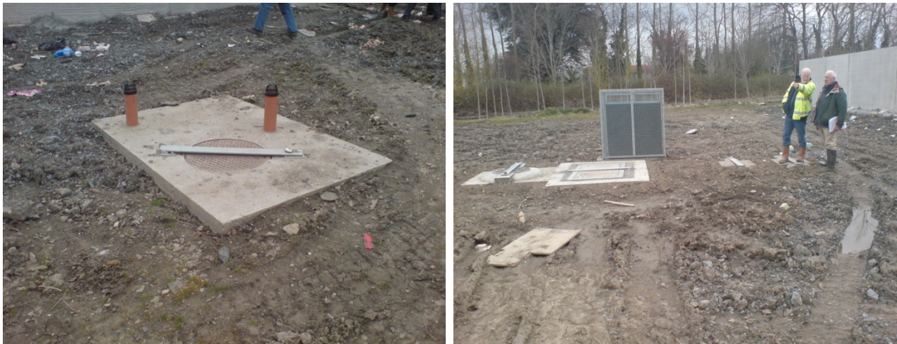
Figure 18 Septic tank and pump sump with control panel
