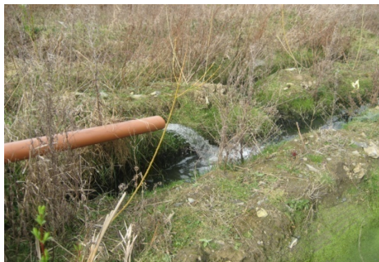
Figure 23 outlet pipe from Horizontal flow bed to willow bed
