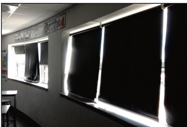
Figure 2: Poorly executed glare control.
