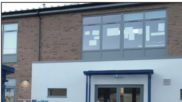
Figure 1: No external shading on south-facing classrooms.
