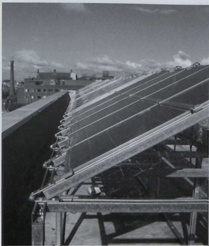
Two parts of the solar energy installation on the roof
