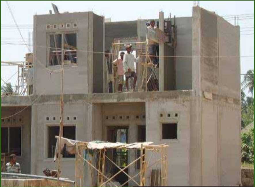
Above: Innovative Slip Form wall construction with team of three unskilled labourers
