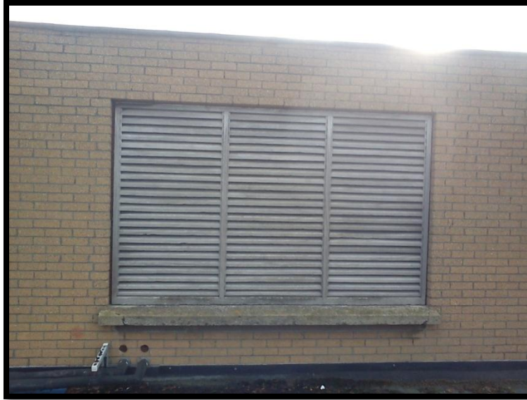
Figure 10: AHU-01 air intake point
