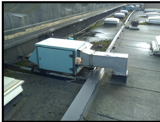
Figure 11: Changing room AHU
