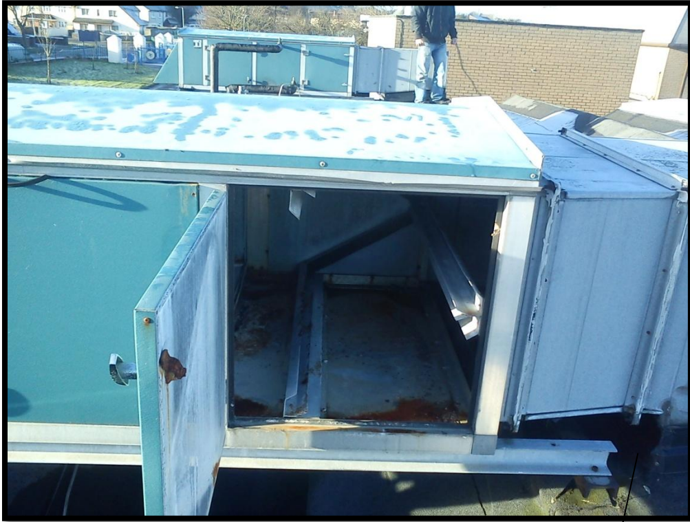
Figure 9: Old extract AHU
