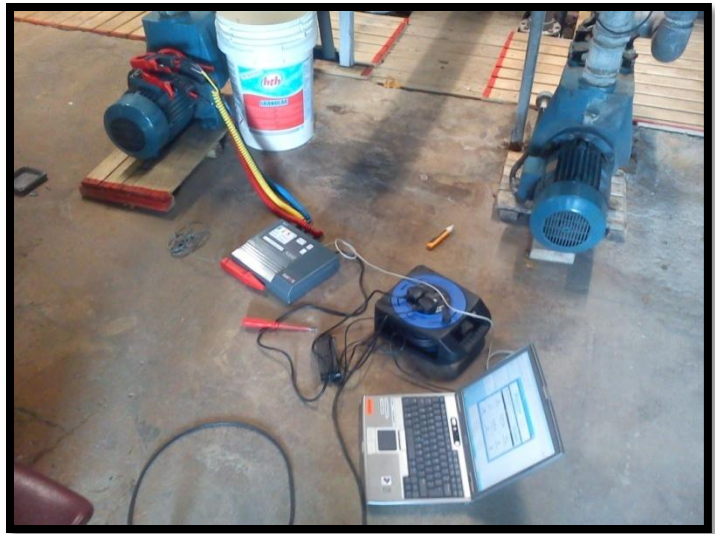
Figure 51: Monitoring the filter motor pumps
