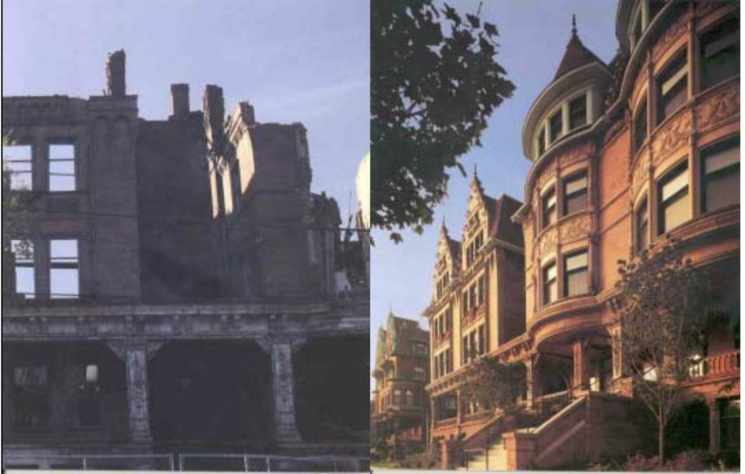
Figures 7A (prior to rehabilitation) and 7B (following rehabilitation): The Brentwood rehabilitation project at Parkside Avenue, Philadelphia. The project involved the rehabilitation of the near derelict Brentwood Building into forty-four residential units for use by low-income families and senior citizens with the assistance of the federal historic rehabilitation tax credit and low-income housing tax credit.
