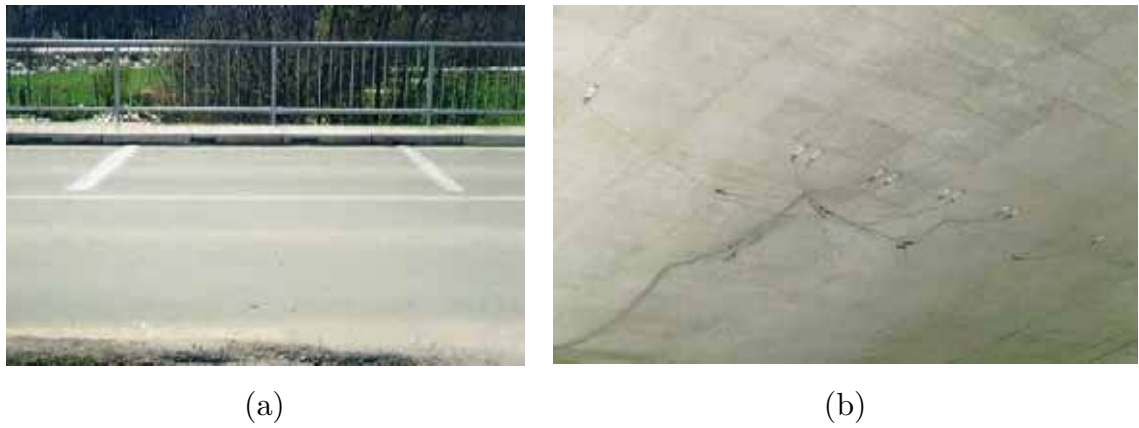
Figure 4.2: WIM installations: (a) road surface axles detectors; (b) bridge soffit strain transducers.
