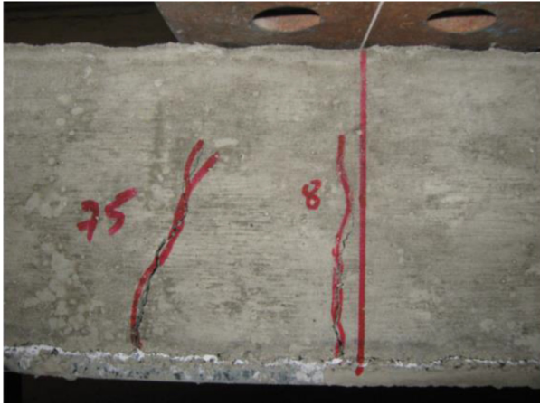
Diagonal Shear cracks – Left hand side
