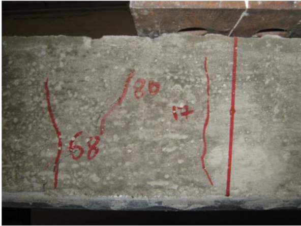
Diagonal Shear cracks – Left hand side
