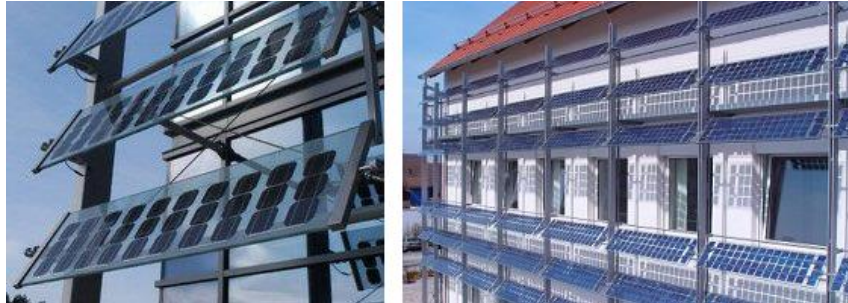
Fig. 5.25 Sun Shades incorporating c-Si Solar Cells [76]
