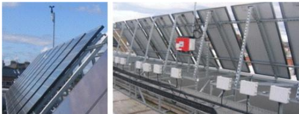
Figure 4.10. The actual solar PV system built and installed at a site in Dublin [121].
