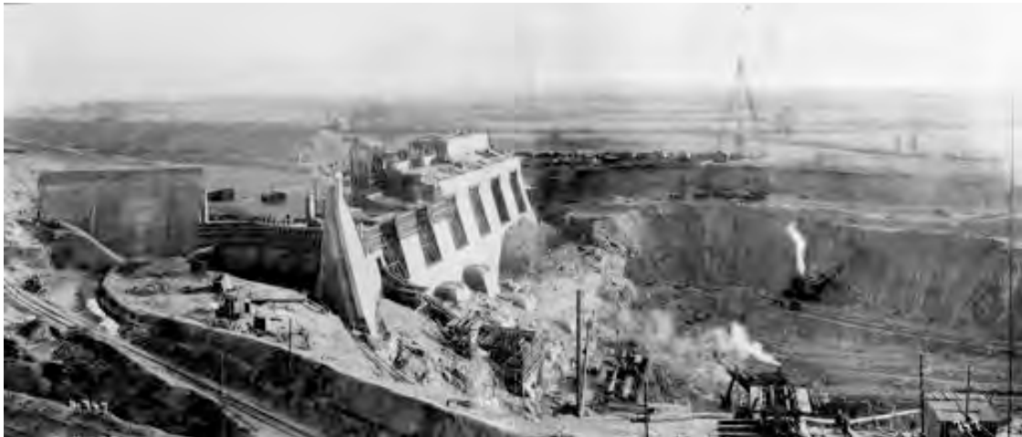
Figure 1.5; 'Power Station, 11 January 1928', Photographer unknown (courtesy Siemens Archive, Munich)
