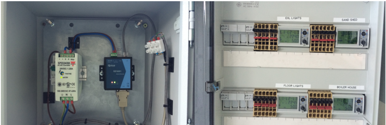
Figure 27: Powersoft Distribution Board
