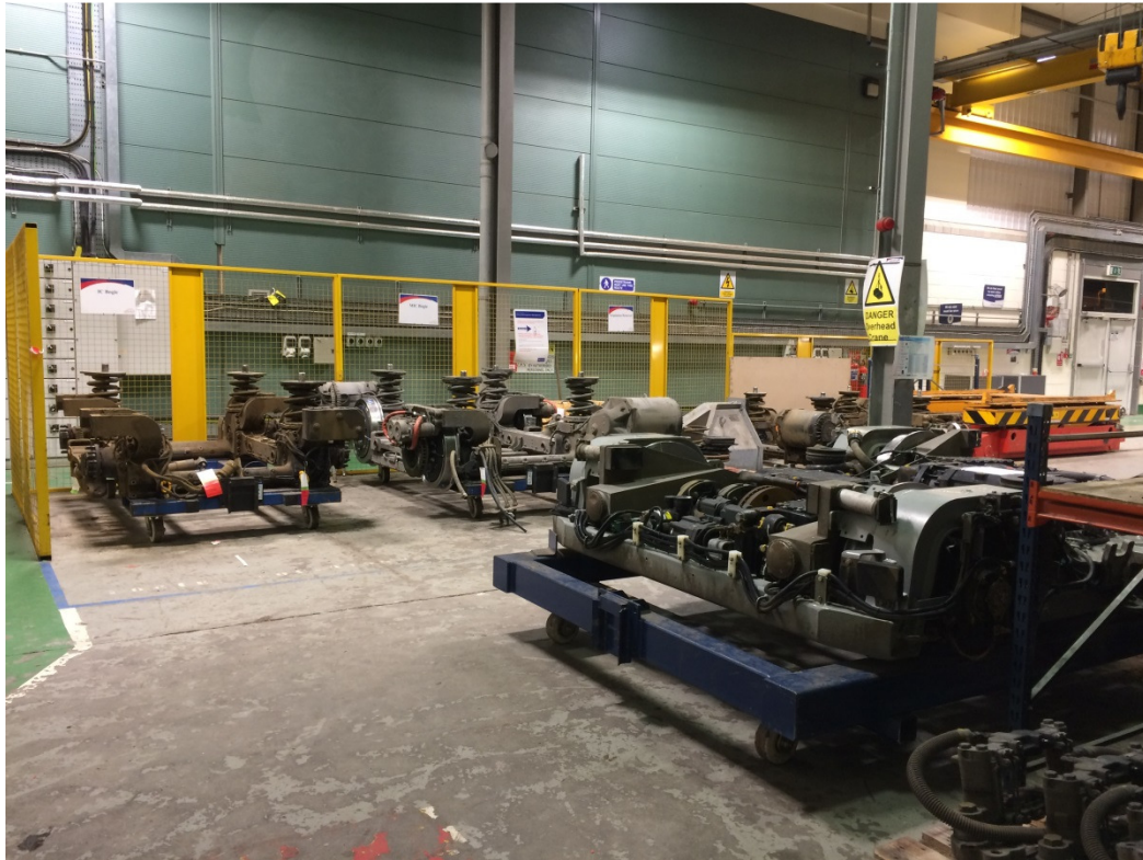
Figure 80: Red Cow Depot Workshop Lighting Trial
