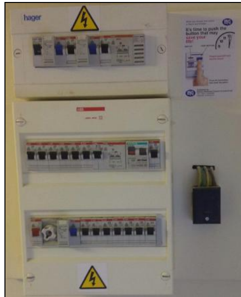
Figure 8.3.7 – 1990's distribution board (consumer unit) with warning label attached
