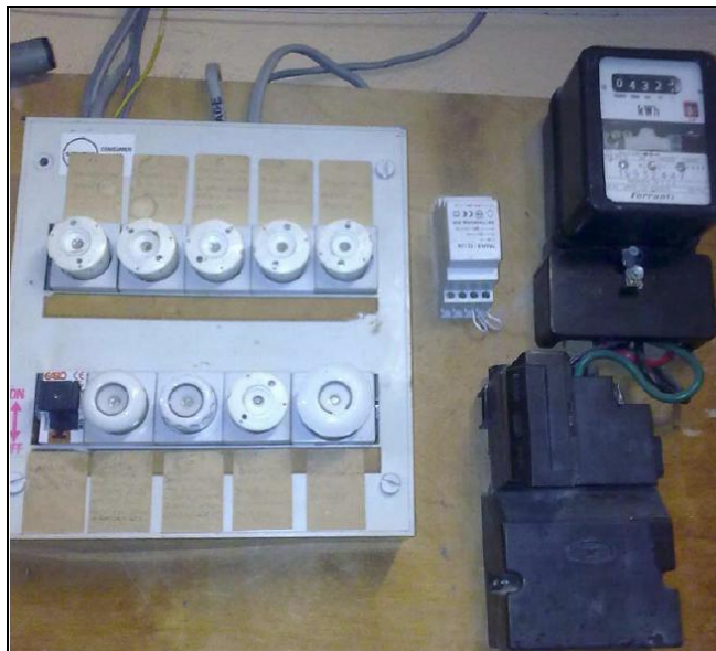
Figure 8.3.3 – Pre 1980's fuse board with service cut-out and metre
