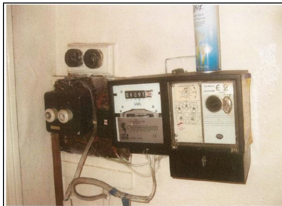
Figure 8.3.1 – Pre 1960's fuse board with coin metre
