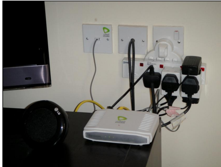
Figure 8.3.10 – Circuit functionality compromised by over load
