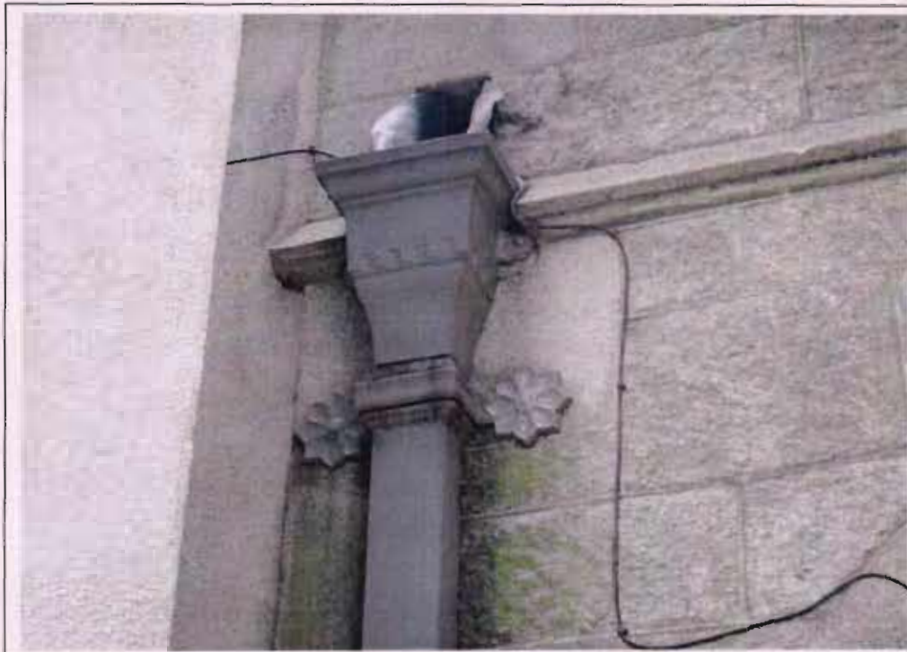
Fig 64: Image illustrating the upper section to the cast-iron down-pipe to the vestry. The suggestion to accommodate telecommunication cabling internally to such piping was suggested by the recorders
