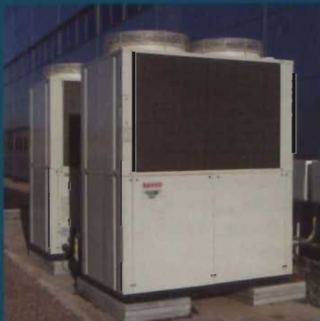
The Sanyo GHP rooftop installation at Citibank, Belfast
