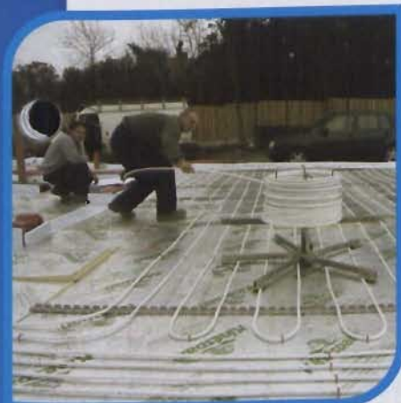
Unipipe underfloor heating
