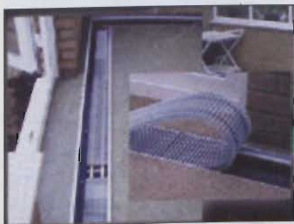
Sill Line perimeter Warmline trench heating
