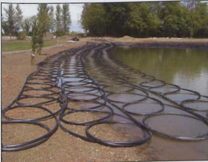
Gathering energy for a large 20,000 sq. ft. house and swimming pool is 8 Kilometres of Uponor Energy Pipe; laid out on the shore initially, floated out onto the lake, then sunk (by plumbers in canoes!)
