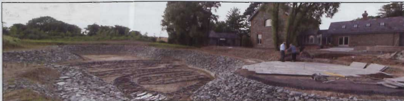
Another Uponor lake collector, this time fitted onto the lake bed before filling; in this instance a fast flowing stream continuously replenishes the heat taken in by the heat pump. The 600m 2 house also has Unipipe floor heating throughout
