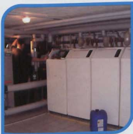
120 kW NIBE Ground Source Heat Pump Installation
