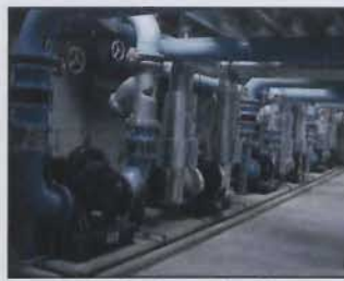
Grundfos horizontal split-case centrifugal chiller pumps for an underground cable ac system in a large industrial park
