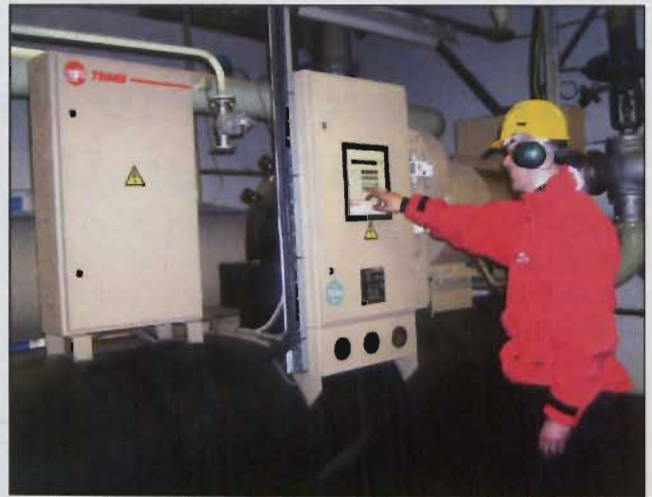
The best form of after-care is a maintenance contract provided by a reputable company employing fully-qualified air conditioning engineers
