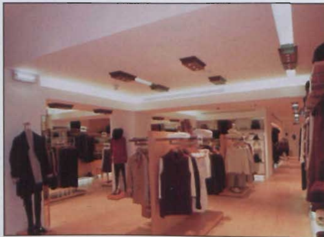
Trane ducted system installed in a retail clothing store
