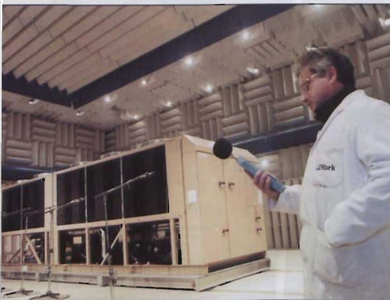
York air cooled chiller in the new York Test Laboratory. The walls are lined with acoustic wedges which create a free field sound environment.
