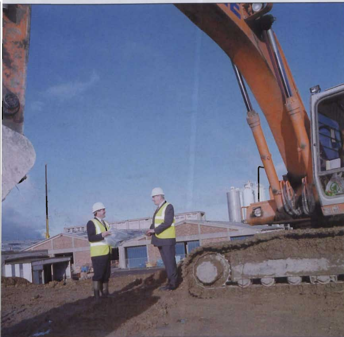
Pictured on the site of the new extension are Fergal McGough, Production Manager (left) and Larry Carr, Managing Director, Wavin Ireland.
