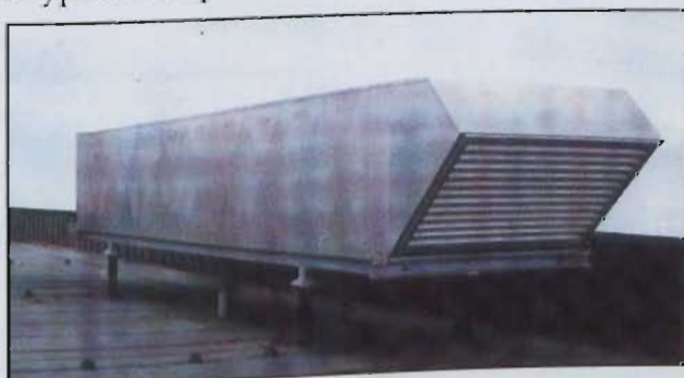
Mark Rooftop air handling unit
