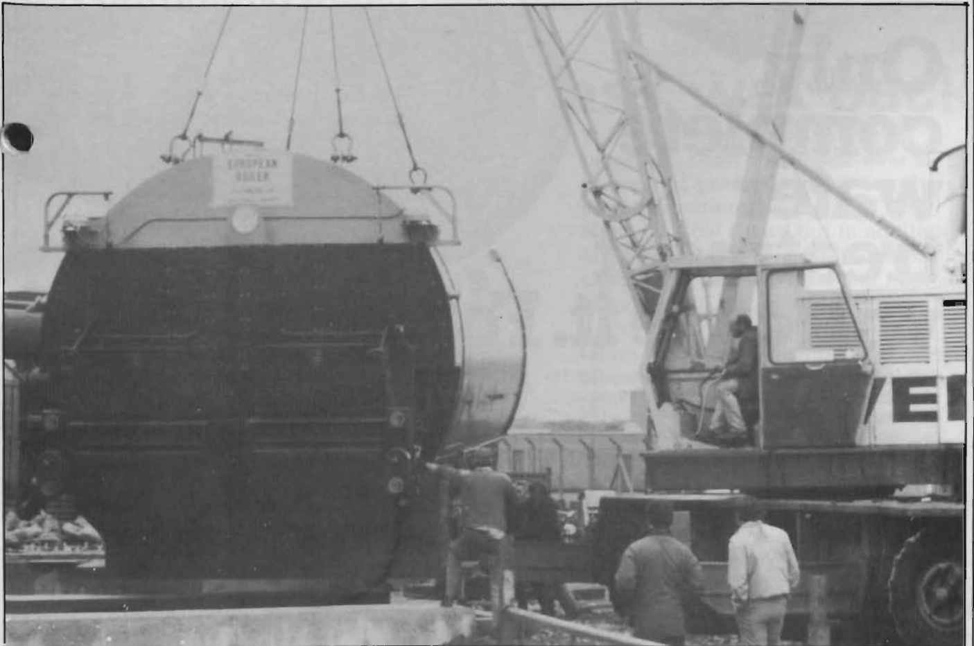
● A twin chain grate coal-fired boiler (25000 lb/hr) being delivered to Canadian Technical Tapes in Bangor, Co Down, prior to installation.
