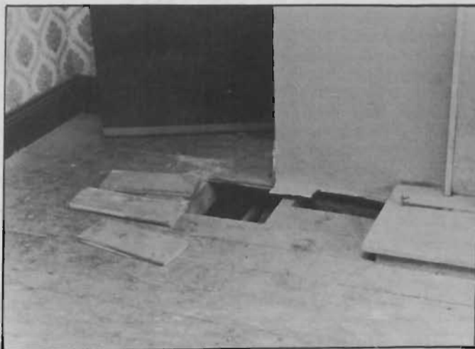
• T & G floorboards in the South Dublin house were simply hacked up.
