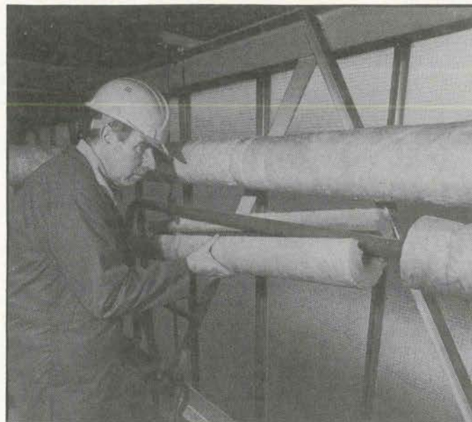
● A lagger snaps Crown Pipe Insulation on to a pipe, where its interlocking Z-lock ensures a tight heat-saving longitudinal seal.
