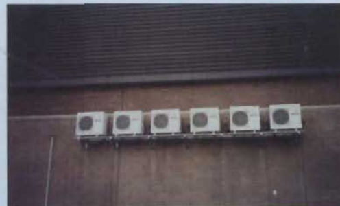
Mitsui heat pump systems (outdoor units) at Abbots Diagnostics, Sligo
