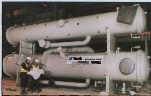
York ACR can provide an infinite variety of refrigeration solutions, be the requirement large or small. Witness to scale of the units above which are part of the refrigeration system devised and installed in the Channel Tunnel
