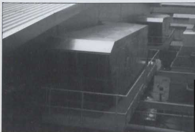
The Mark Eire external gas AHU's at the Shelbourne Hall, RDS.
