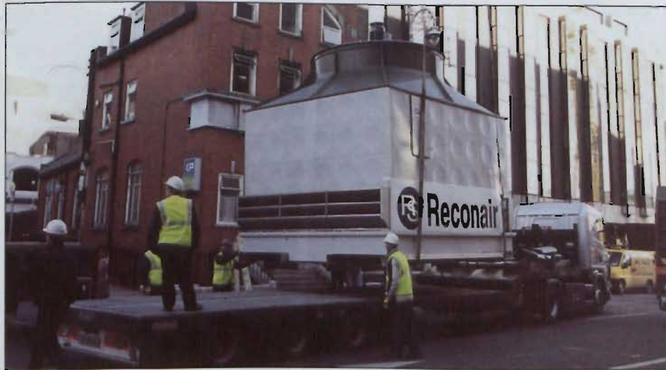
Irish Life is one of Reconair's many blue-chip clients. Just recently the company completed a massive project in Abbey Street which brought Dublin to a standstill (see BSNews October/November)
