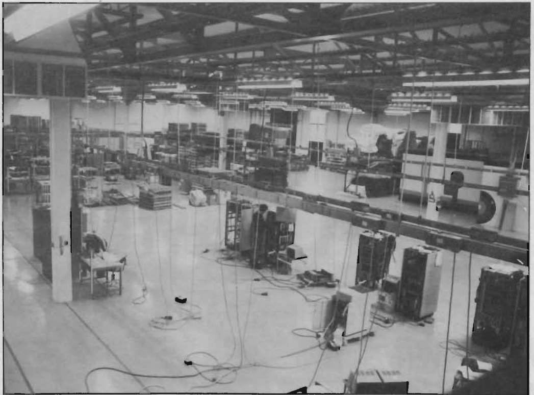
● Five Carlyle 50DF series packaged cooling units supplied by Walker Air Conditioning have been installed on the roof of the Modcomp computer factory in Carrigtwohill, Co Cork. Although originally installed as insurance against possible heat damage, operating conditions in the factory have, to date, caused the cooling units to prove their worth mostly in terms of the essential comfort conditioning which they also provide.
