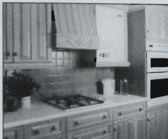
Right: Typical Keston condensing boiler installation
