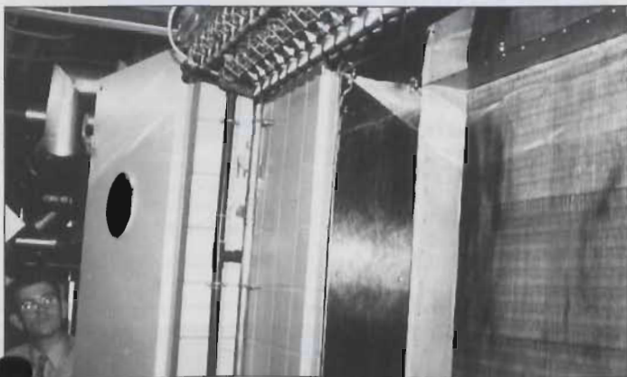
JS JetSpray in-duct nozzles provide safe humidification for 180,000 sq ft at Midland Bank. An engineer checks out the new humidification manifolds in an existing AHU.
