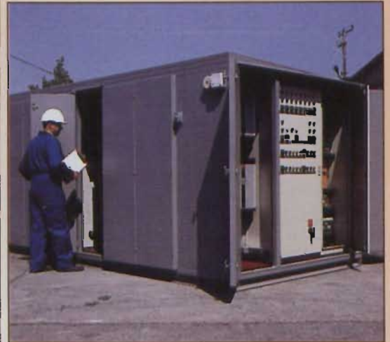
Final commissioning check on packaged boiler house prior to client hand-over
