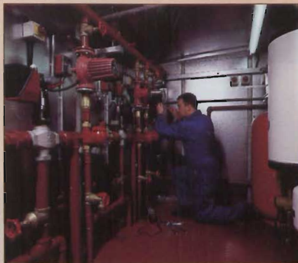
Packaged boilerhouse being pre-piped and pre-wired with TAC controls
