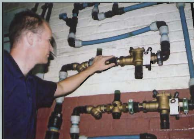
Honeywell back-flow prevention valves installed at Ralken Colours
