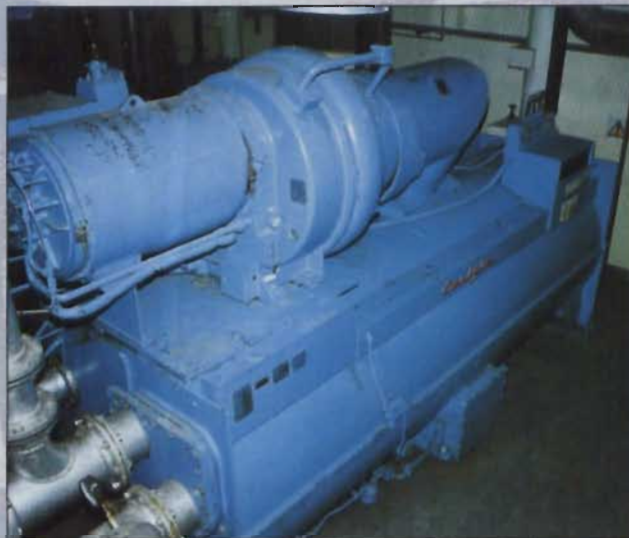
The in-situ Carrier chiller before work commenced
