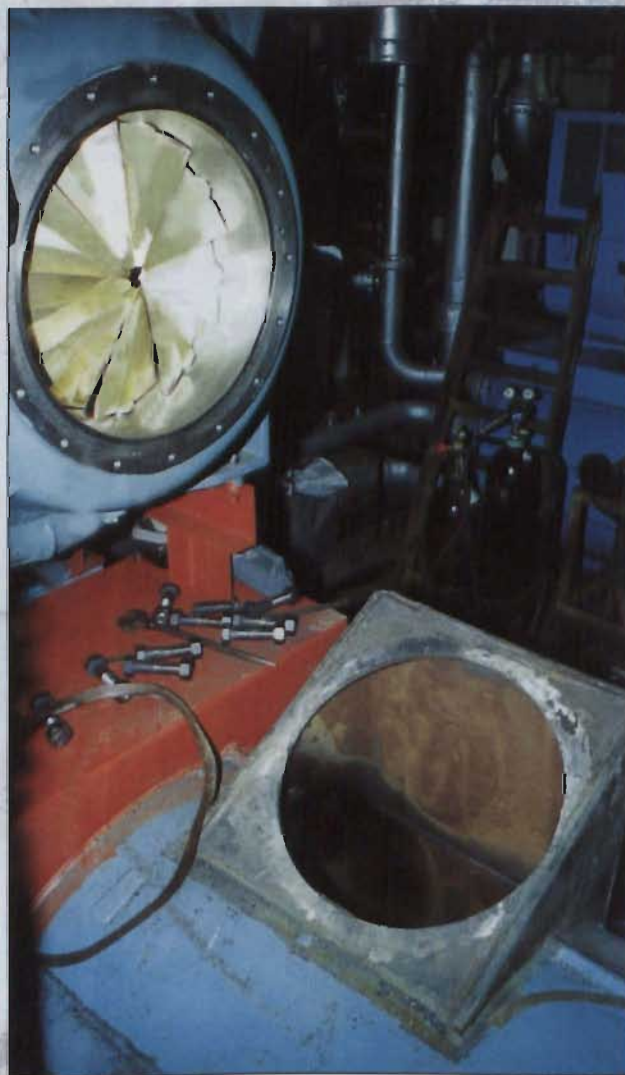
The suction connection prepared for new suction elbow
