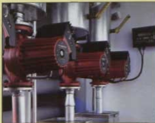
Below: Heating installation using three Grundfos UPE 32-120 units from the PMU 2000 range
