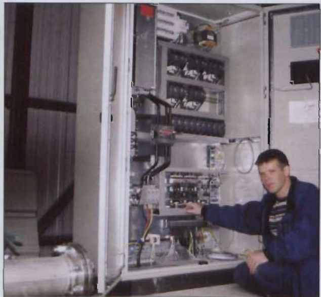
Kevin Sullivan, Wilo service engineer, commissioning the controls of the new Wilo booster set
