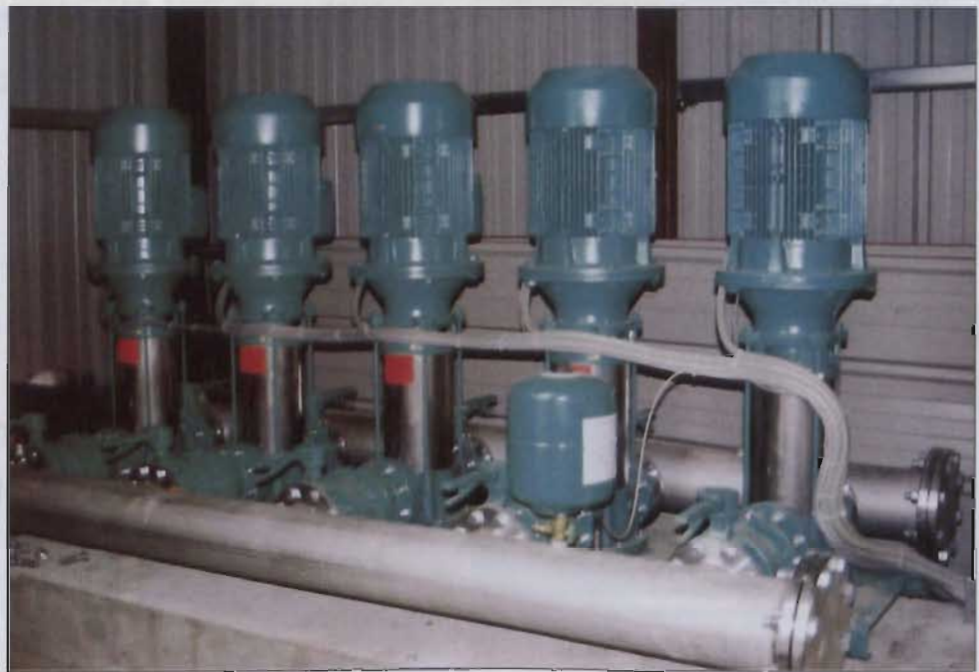
The new Wilo booster set recently installed at Ballymun Regeneration Project
