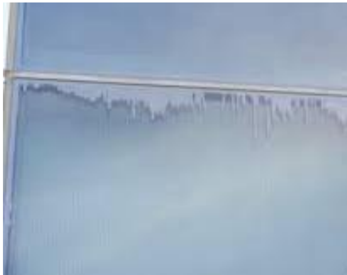
Figure 5.1 Migration of a PIB sealant into the vision area of an IGU
