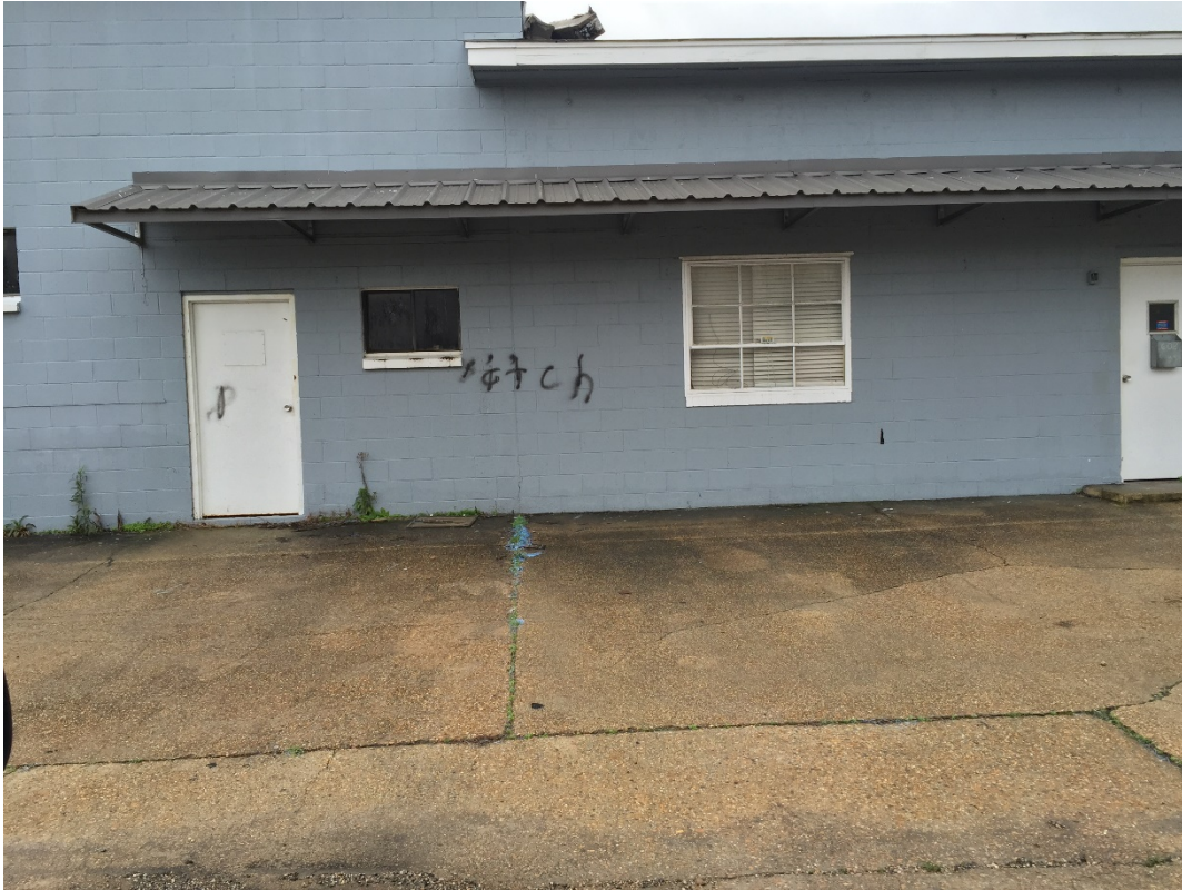
Figure 12. Abandoned Building with Graffiti on East 7 th Street along Route 3 (Photo by author).
