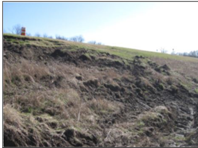
Figure 2. Slough or slump slide on a levee.
