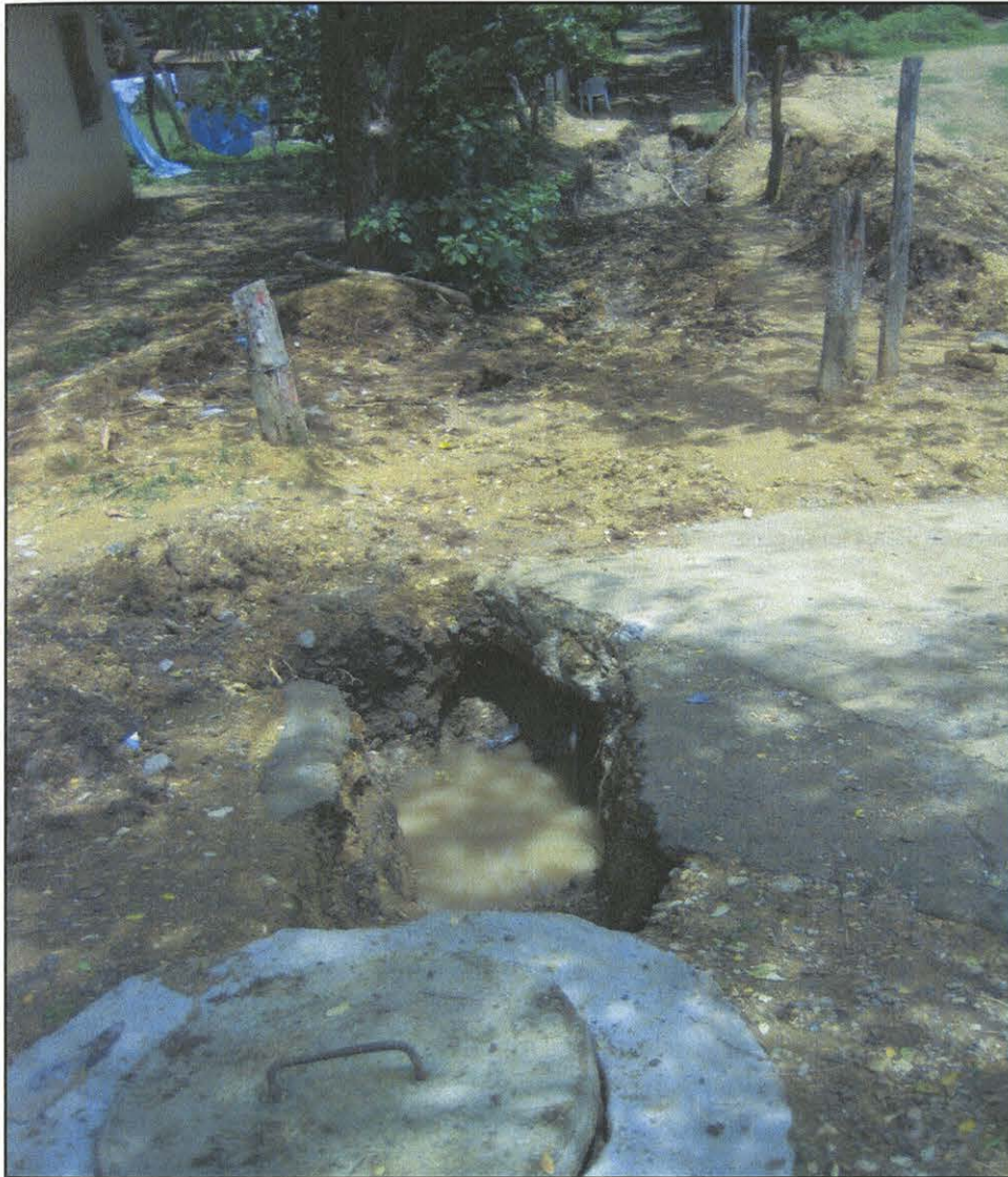
Figure 21. Unfinished Sewer Project in Jose Alberto Barbarena.
