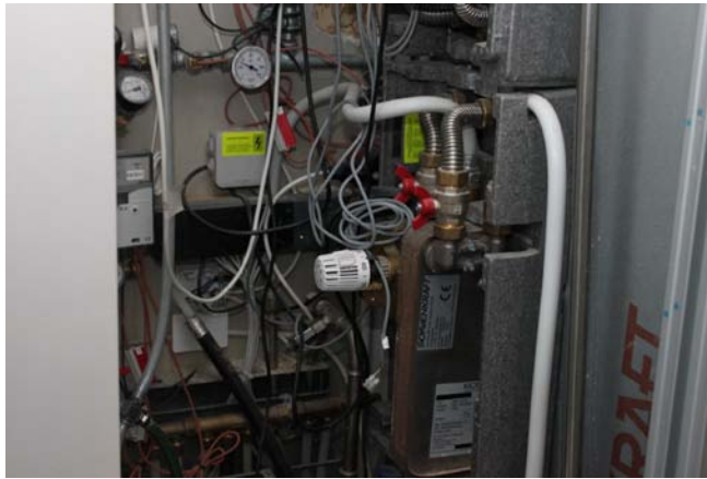
Figure 13: Heat exchanger inside the house
