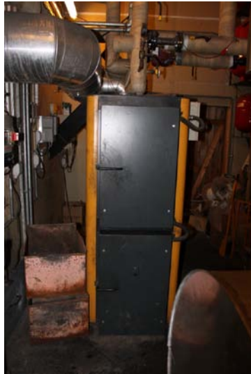
Figure 2: Granules boiler (180kW)
