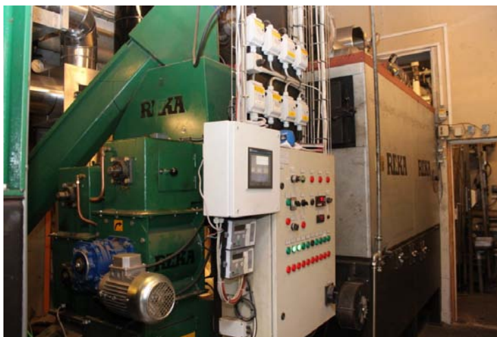
Figure 4: Central wood chip stove ( 160kW)
